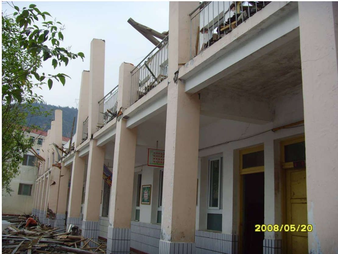
Damaged building in BeiChuan 2008-5-12-14:28
