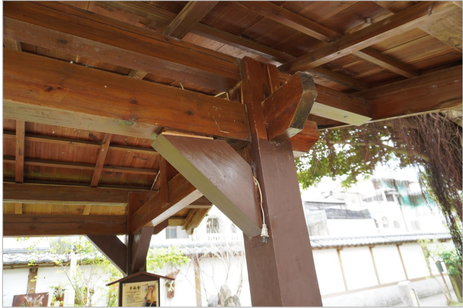
Figure 48 J4 手水舎の被害
