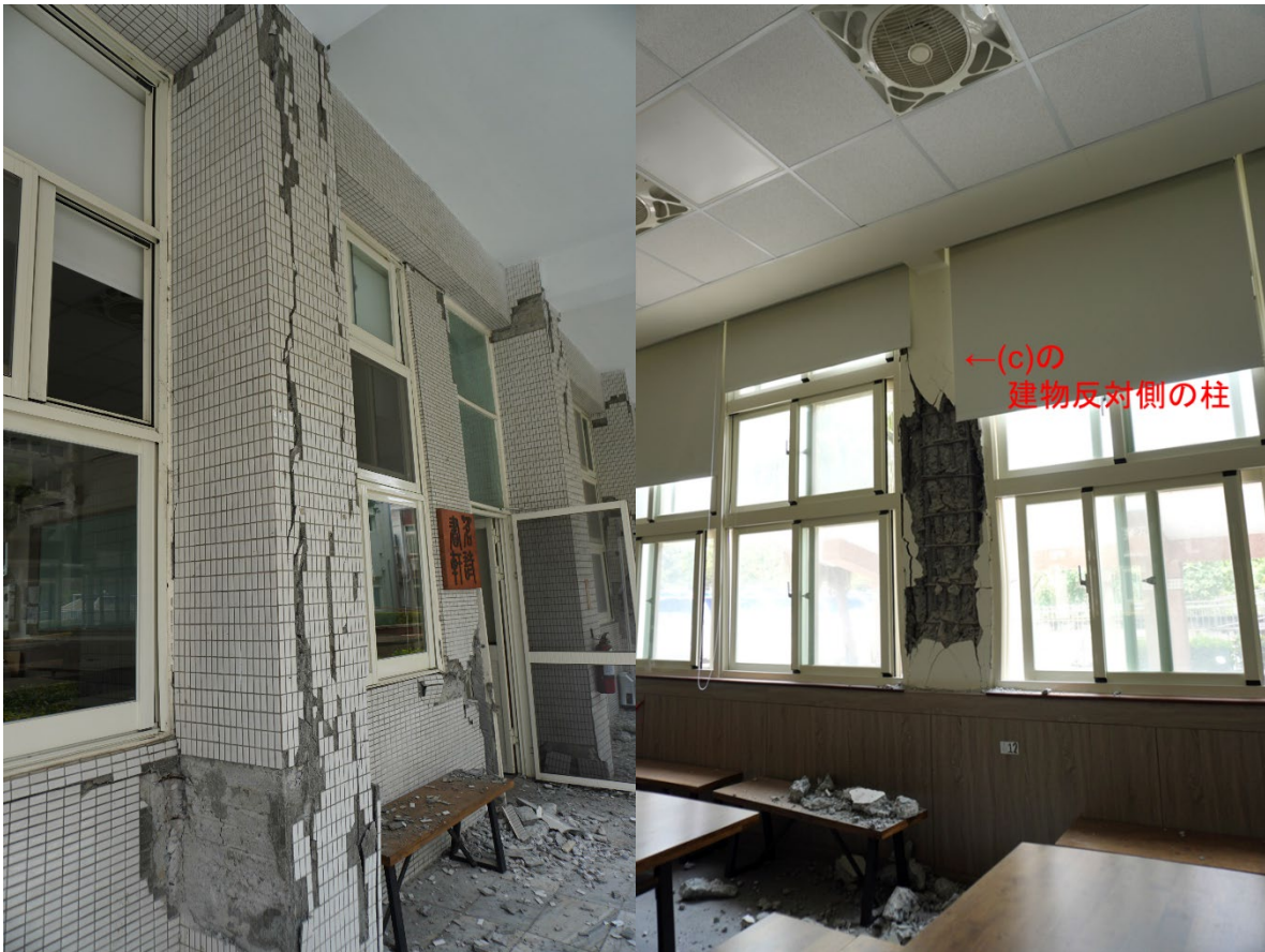
(c) 柱の付着割裂破壊
